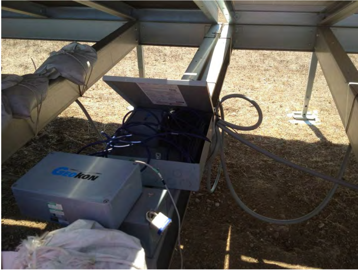
Photo 3: Geokon Data Logger Model 8002-4-2
